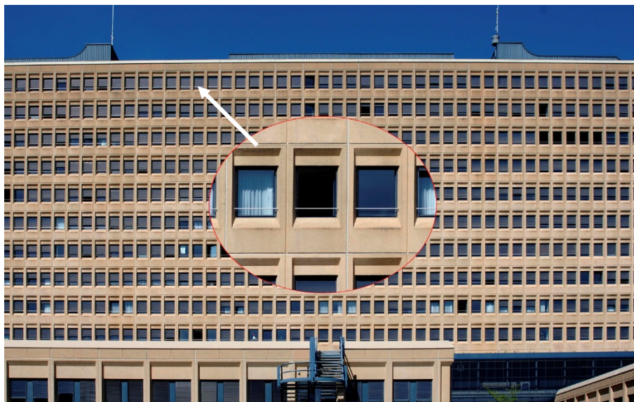
Figure 1 The metal rail installed at each of the 1'240 hospital windows.
